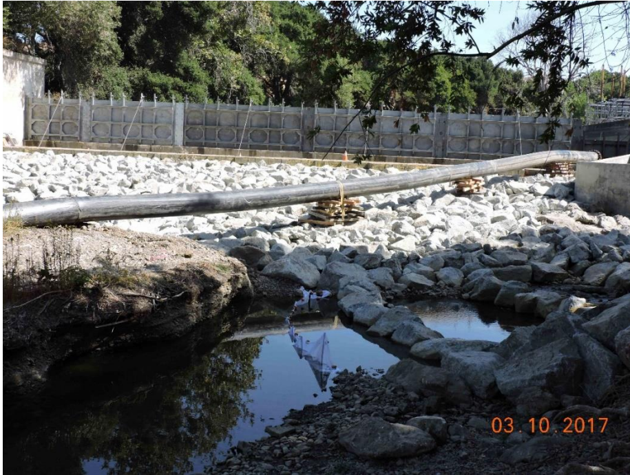
Photo 7. Metcalf Pond dam panels reinstalled and dam apron buttressed with grouted boulders on 3 October 2017. Flow bypassed in pipeline to allow grouted boulder weir construction that was necessitated by channel down-cutting during flood.
