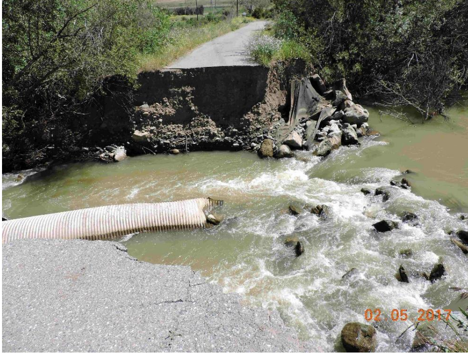
Photo 16. Washed out road and culvert immediately downstream of Ogier Pond #1 on 2 May 2017 at approximately 150 cfs. Stream flow was still turbid (16 cm visibility) from storm water stored in Anderson Reservoir. Visibility had cleared to 75 cm by 26 October 2017.
