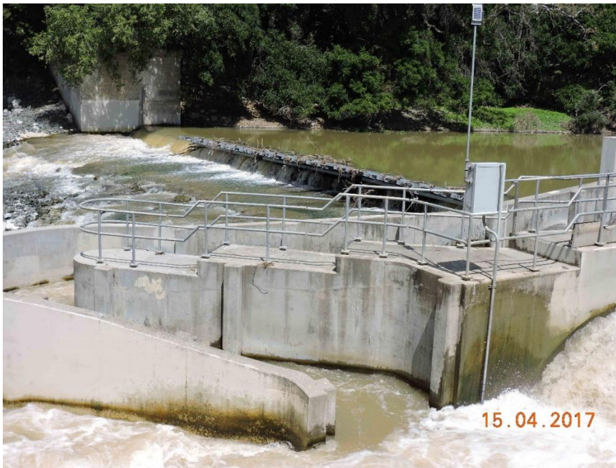
Photo 6. Metcalfe Pond Dam on 15 April 2017, with a functioning fish ladder that had been modified for passage by 30 March.
