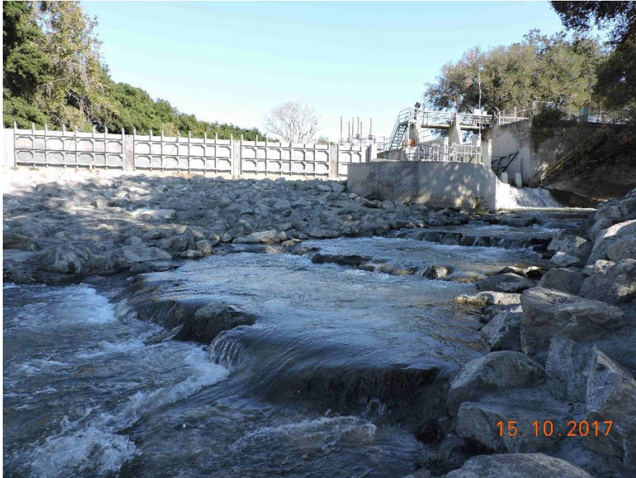
Photo 9. Grouted boulder weirs on 15 October 2017, with pipeline removed and flow through radial gates. Gates were slowly closed (to maintain a live stream downstream) raising the Metcalf Pond water level, and allowing flow to spill through the fish ladder 1 week later.
