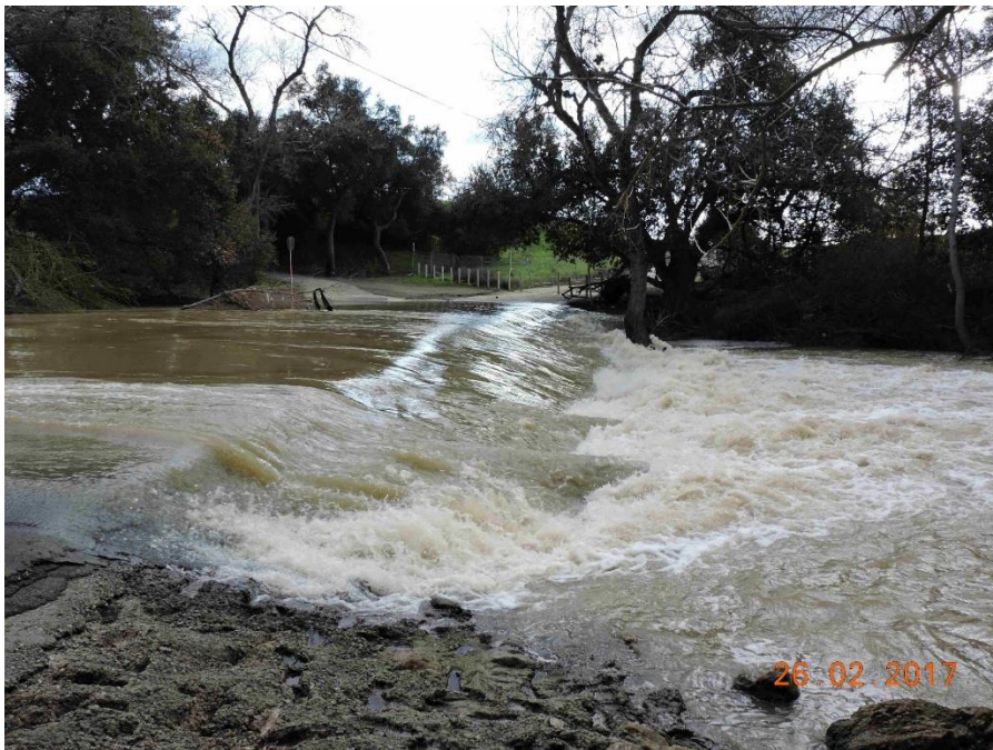
Photo 10. Singleton Road on 26 February 2017 at 650++ cfs, with no adult steelhead passage possible because of high velocity in the two submerged culverts and on the steeply inclined apron.
